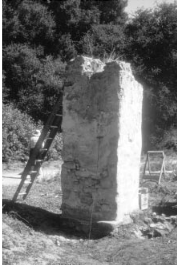
Fig. 5. Single standing column of brick, stone, tile fragments, and cement is all that remains above ground of the possible windmill foundations at La Purísima.
